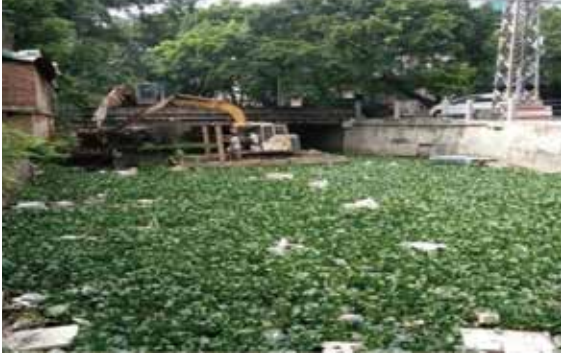
Black and odorous water before treatment 黑臭水體治理前
